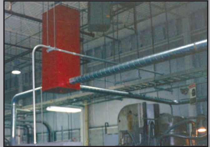
OM3510 Oil Mist Multidrop-ducted to three CNC lathes.
