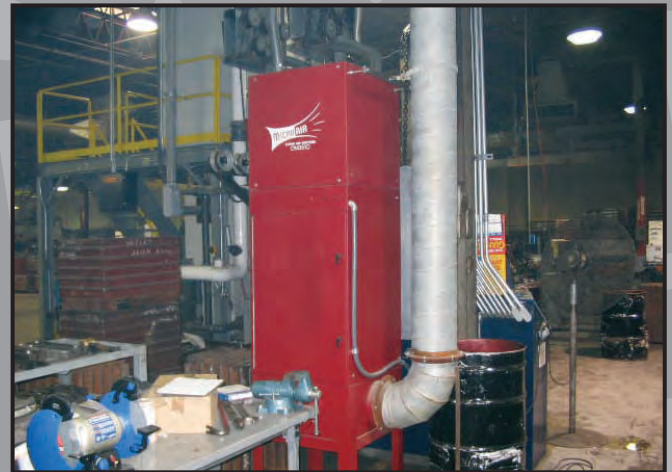
OM3510 ducted to lathe.
