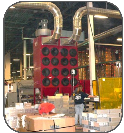
RP8-2 with Ducted to Multiple Weld Cells in Aluminum Mailbox Manufacturing Facility
