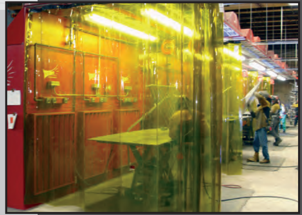
Multiple Clean Air Booths with Regain Air in Welding/Grinding Operation
