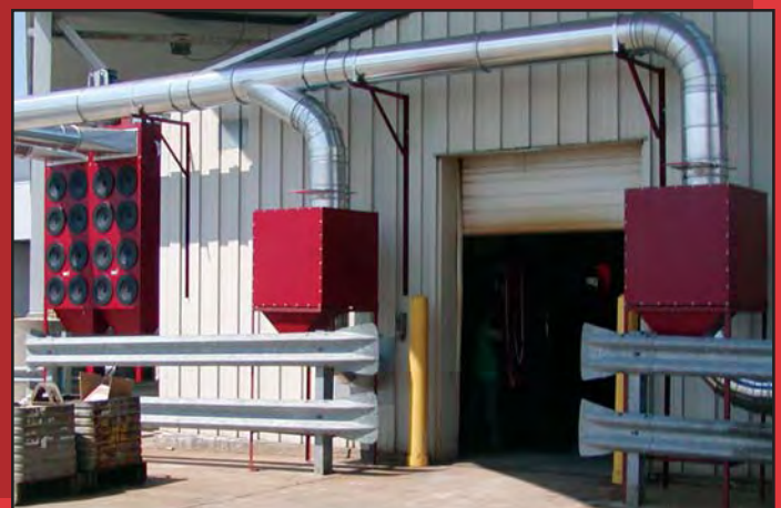
RP8-2 with spark arrestors collects laser smoke.
