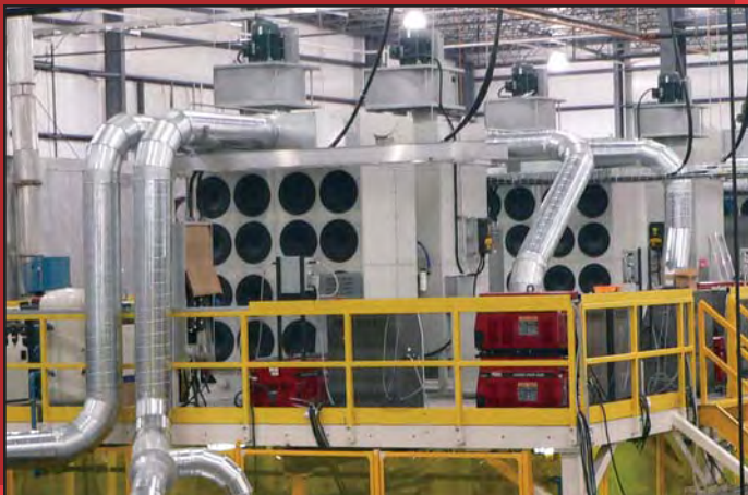
RP8-2 Collects Smoke/Fumes from Robotic Weld Cell
